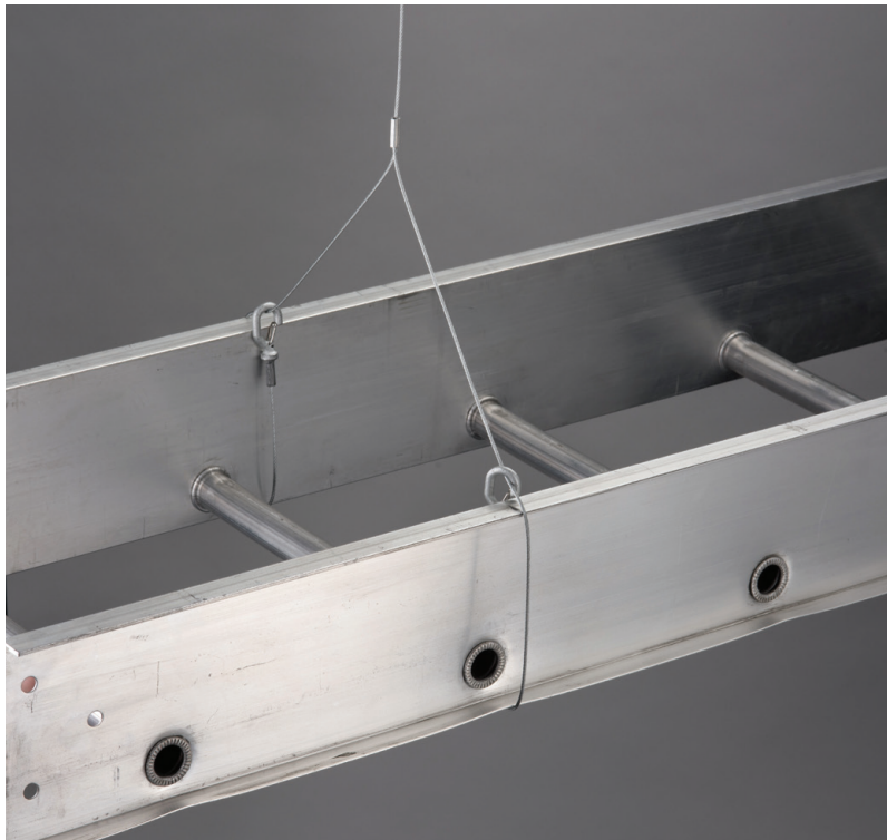
Figure 3: Speed Link SLK with Y-Hook supporting a cable ladder
