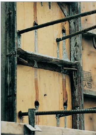
Drilling forms for dowels is expensive, and form removal is difficult and time consuming.
