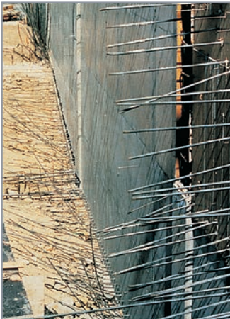
Exposed dowels on the job site are a hazard. In addition, they can be bent or damaged.
